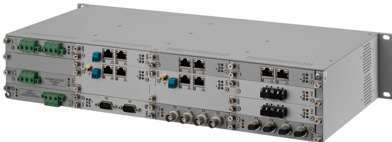
Rear view of base system FG8201G02 with redundant power supplies (n+1 configuration) FG8901P01 / FG8901P06, management controller board FG8800M00, redundant Rubidium time domain controller boards FG8701G01 and service provider boards FG8801N02, FG8801F02, FG8802S01, FG8802S20 and FG8803S02
